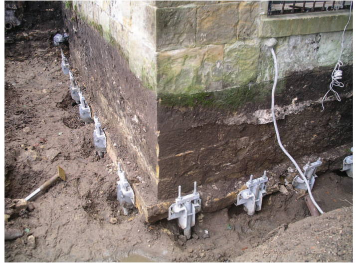
FIGURE 10. CORNER OF FOREST LODGE GATE HOUSE AFTER INSTALLATION OF SCREW-PILES AND FOUNDATION BRACKETS.
